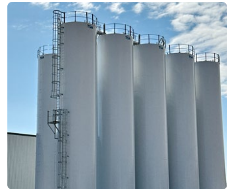
Silos have been erected and the piping for material handling is progressing as planned.
