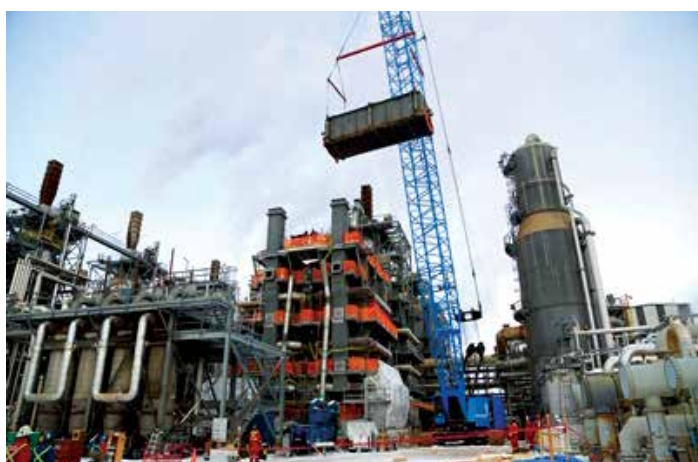
A recent project milestone was the removal of the last large piece of equipment in the refurbishment of the first furnace.
